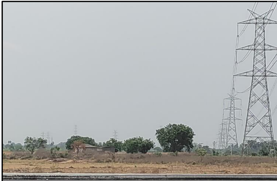
400 kV Transmission Line
