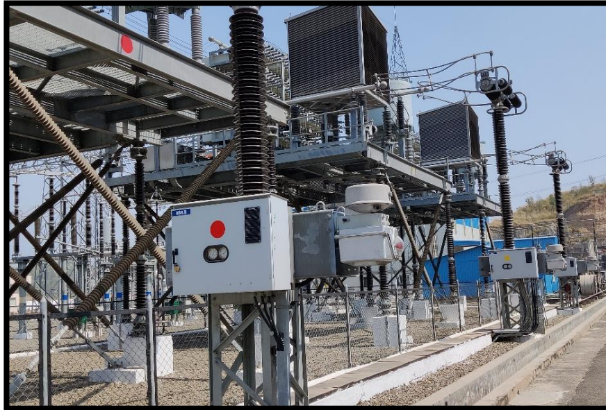
Fixed Series Capacitor
