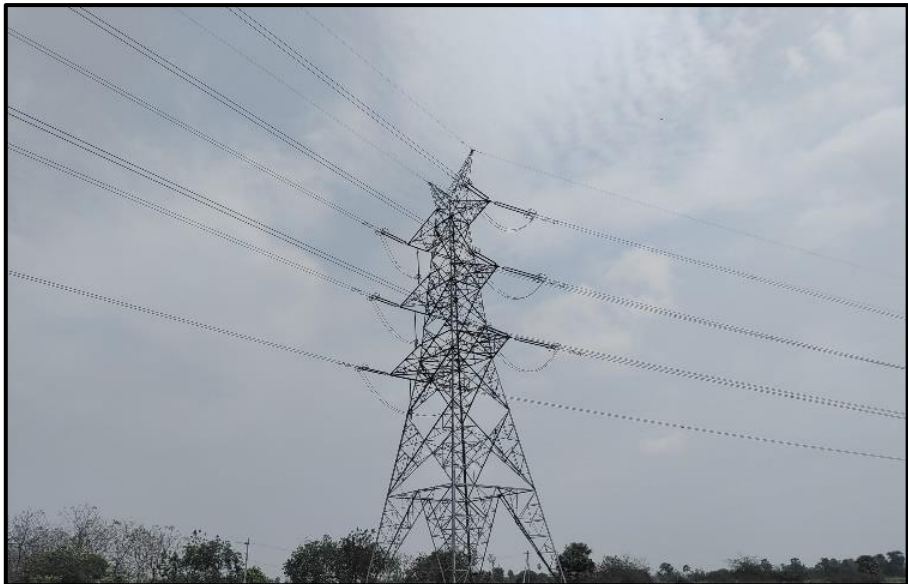
Angle Tower of 400 kV Transmission Line
