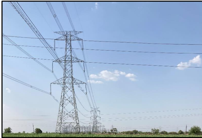
Transmission Line – 400 kV Parli (New) – Parli (PG) Line
