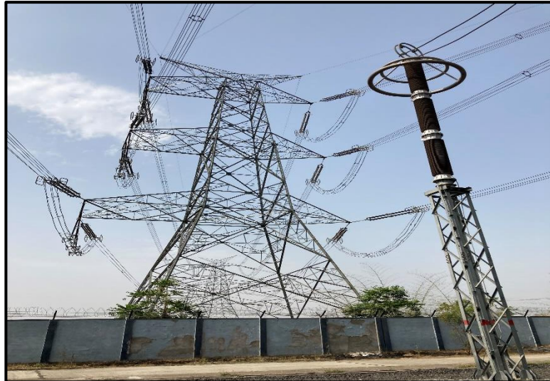
765 kV D/C Vindhyachal Pooling Station- Jabalpur Pooling Station line entrance at POWERGRID Jabalpur Substation
