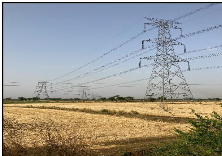
765 kV D/C Vindhyachal Pooling Station- Jabalpur Pooling Station line
