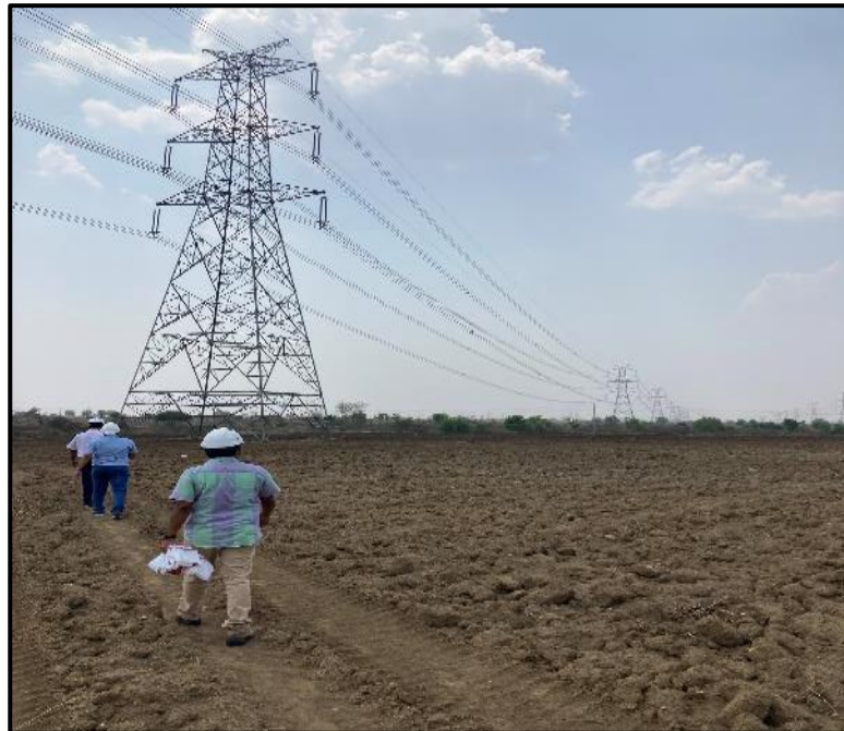
Transmission Line – 765 kV Warora (Pooling Station) – Parli (New) Line
