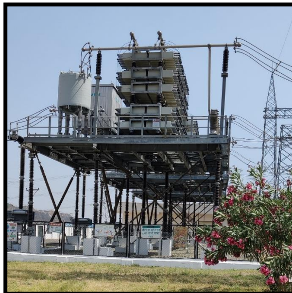
Fixed Series Capacitor
