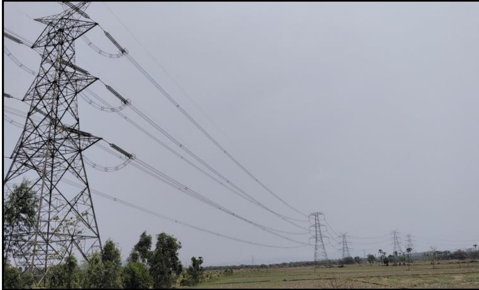
Angle Tower of 765 kV Transmission Line
