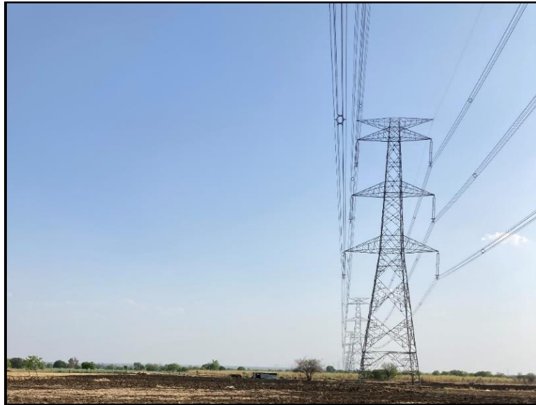
Transmission Line - 765 kV Parli (New) – Solapur Line
