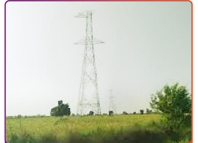
765kV Ghatampur TPS-Agra SC line
