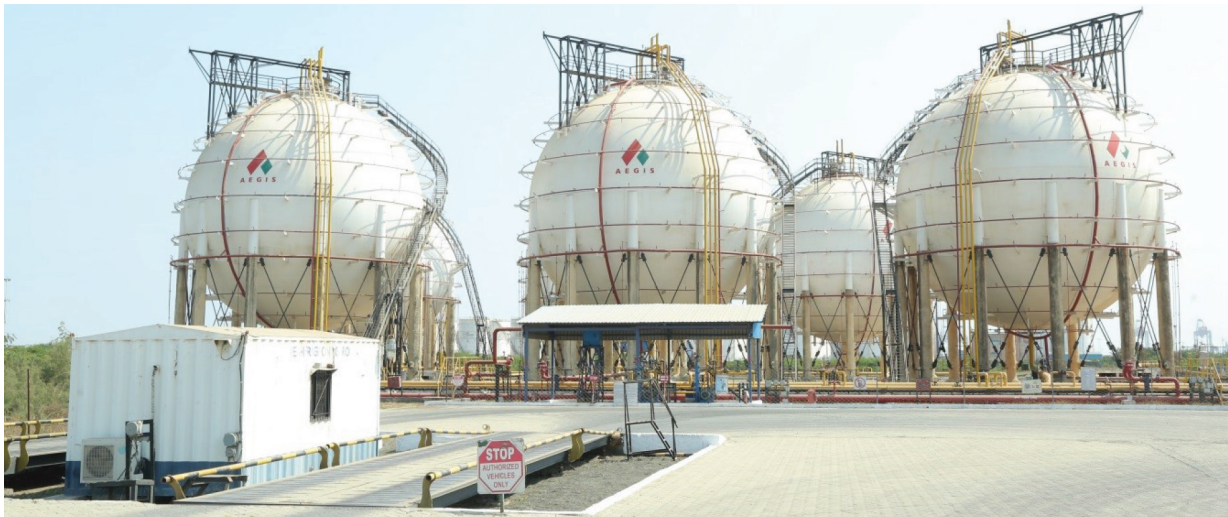
Pipavav LPG Terminal
