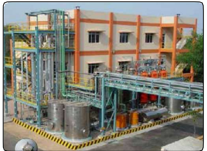
A section of the Fine Chemicals Plant
