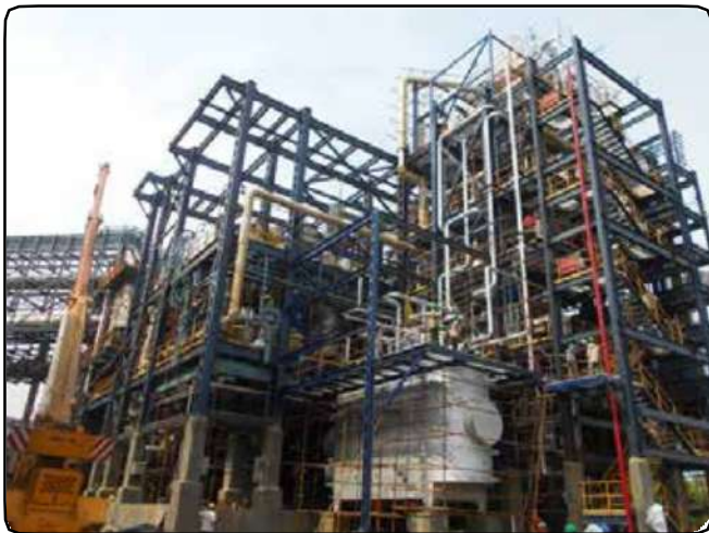
PA Plant Revamp : Oxidation Section - Ranipet
