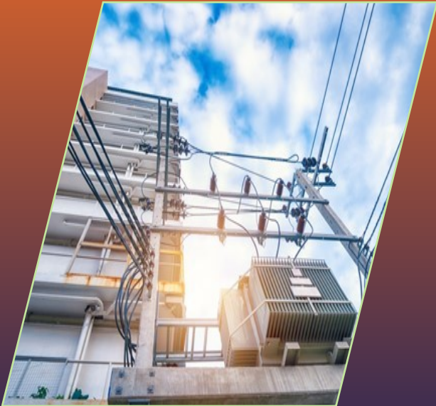
Urban and Remote Transformers
