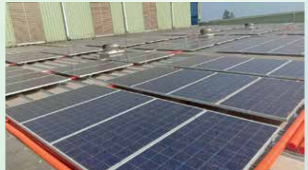
Solar Installation at Stampings, Zaheerabad plant
