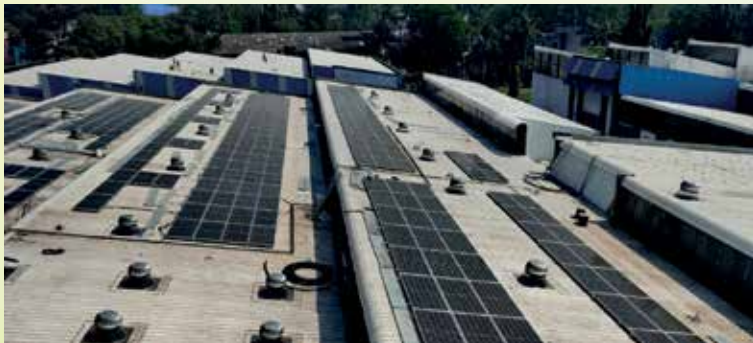
Solar Installation at Magnetics, Bhosari
