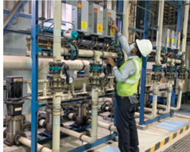
Energy conservation with VFD
