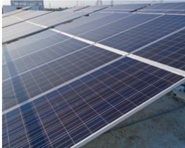
Rooftop Solar for captive consumption
