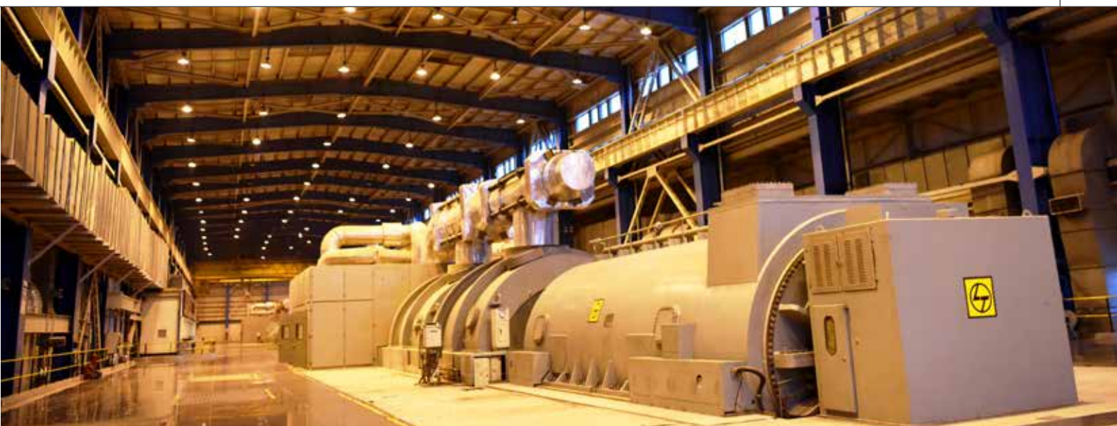
Turbine Generator at Nabha Power Plant, Rajpura, Punjab
