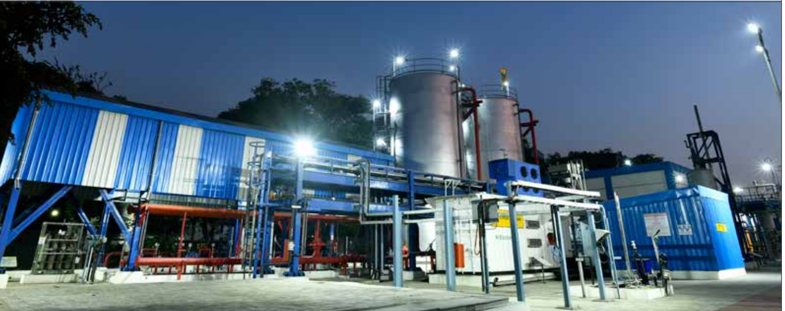
Green Hydrogen Plant at L&T's A.M. Naik Heavy Engineering Complex in Hazira, Gujarat
