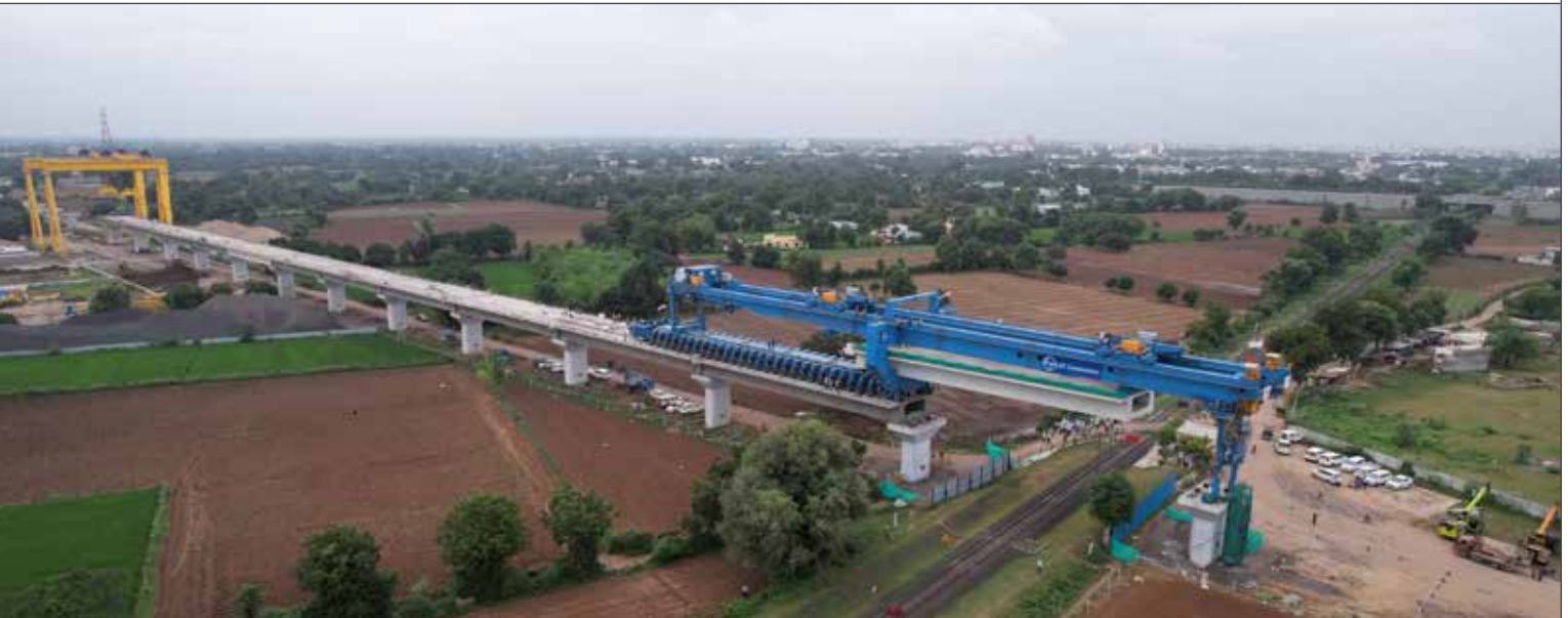
Indigenously designed and manufactured Full Span Launching Machines for Mumbai-Ahmedabad High-Speed Rail (MAHSR)
