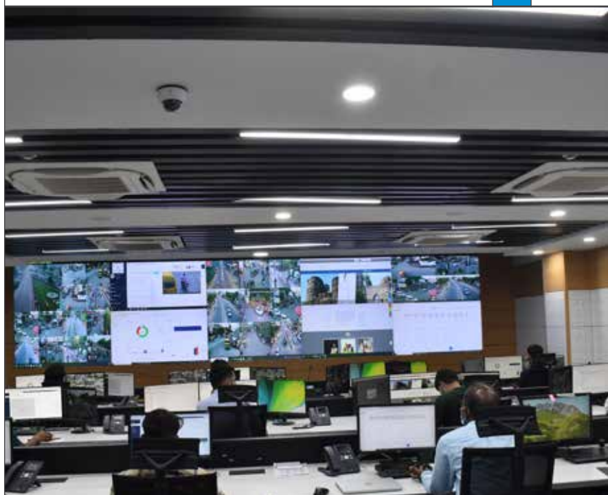
Jhansi Smart City Command and Control Centre
