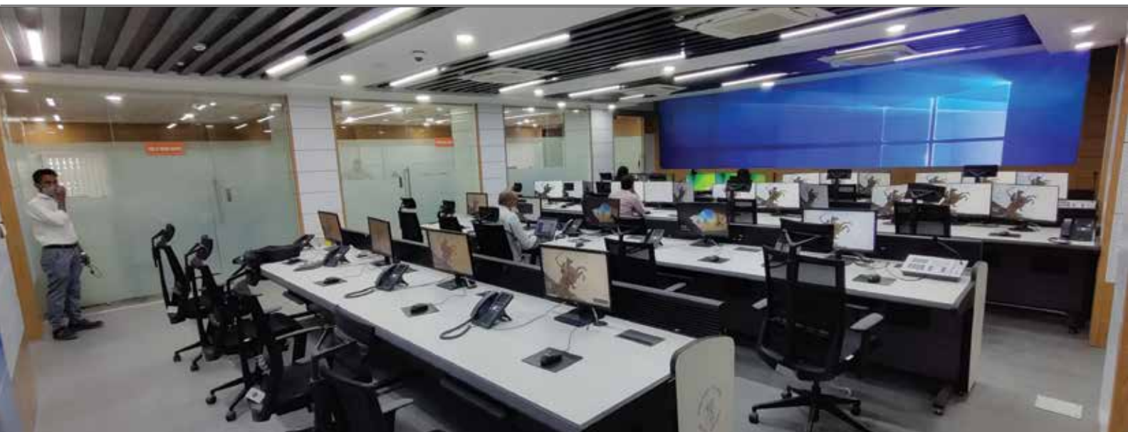
Control and Command Centre, Jhansi Smart City
