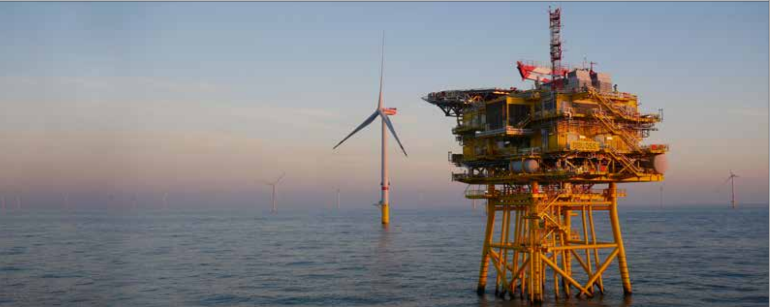
Offshore substation platform
