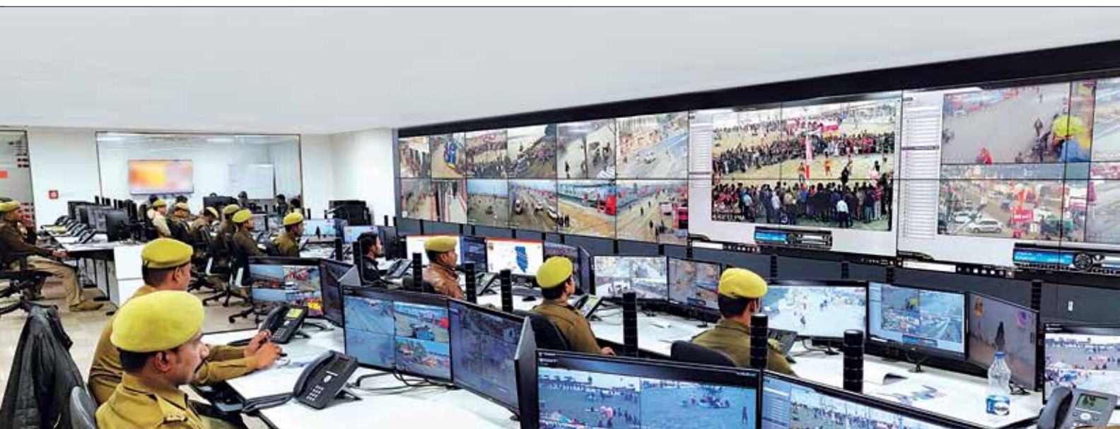
Command and Control Centre, Prayagraj Smart City
