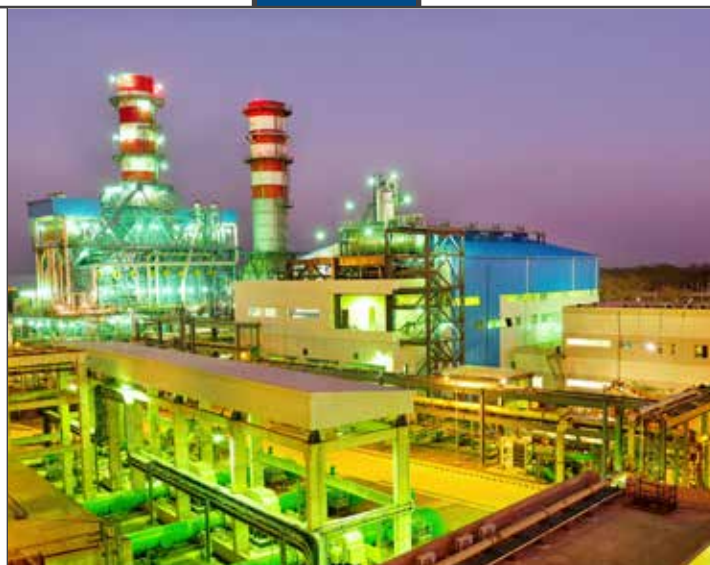
Sikalaha Combined Cycle Power Plant, Bangladesh
