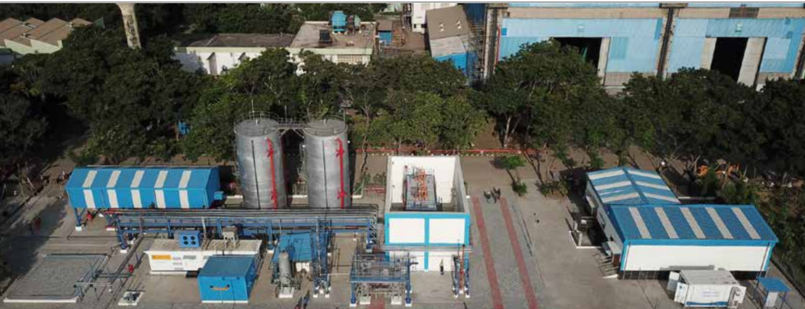
Green Hydrogen Plant at L&T's A.M. Naik Heavy Engineering Complex in Hazira, Gujarat
