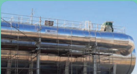
4.3 MLD Zero Liquid Discharge Plant Jagdalpur, Chhattisgarh, India The largest central zero liquid discharge plant of steel industry in India
