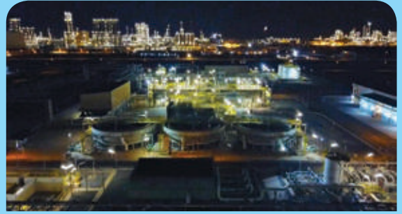
Industrial Effluent Treatment Plant for PETRONAS Johor Bahru, Malaysia One of the largest Effluent Treatment Plant in South East Asia
