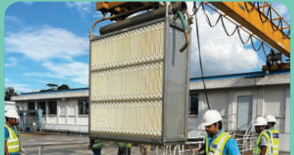
Ceramic membrane plant - 300 MLD Chestnut Waterworks, Singapore One of the key reference for WABAG in the field of ceramic membranes
