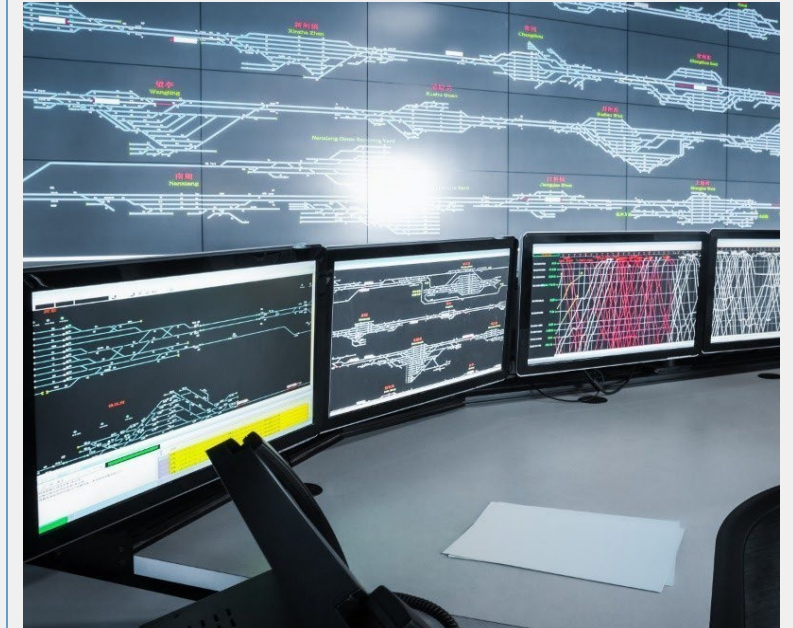
Implementing IP based Video surveillance system (VSS) for railways
