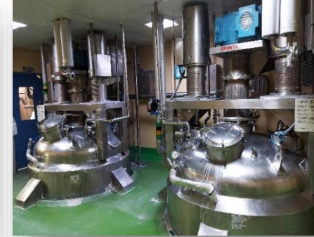
Main Mixing Tank
