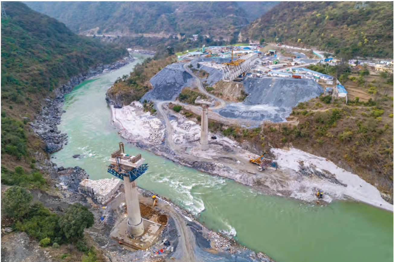
Successful completion of substructure works of Rail Bridge no 8 in connection with ongoing new BG Rail Line Rishikesh- Karnaprayag Project https://youtube/AwXC04aL89s
