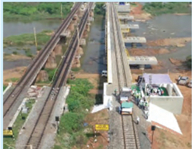
Commissioning of 3rd line between Talamanchi and Srivenkatewarapalem in Vijayawada Division of South Central Railway on 24.12.2021
