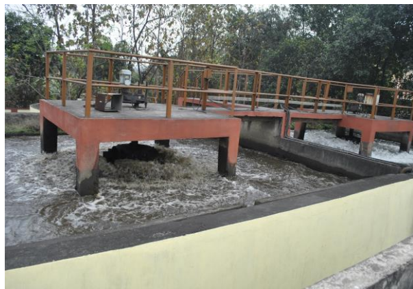
Fig. 50 - STP in Ananta OCP of MCL
