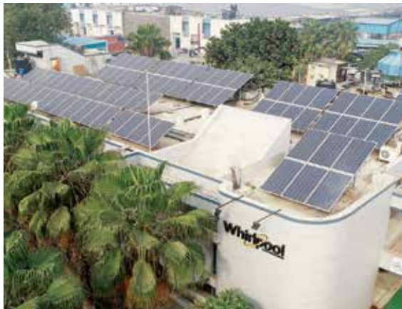
Solar panels installed at Faridabad factory
