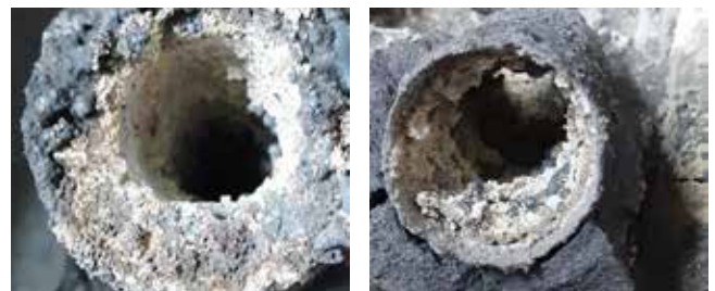
Typical Clogging Occurred
