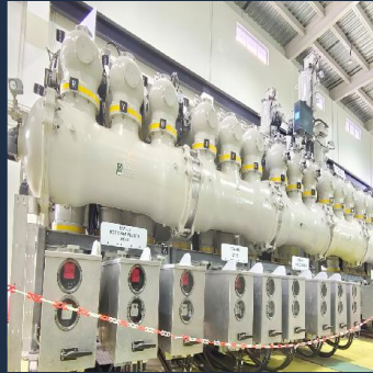
220/110kV GIS substation for KSEB at Ettumanoor
