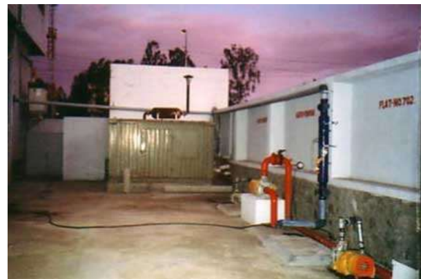
Saving 65.0 lakhs liters of ground water through water harvesting facilities at units
