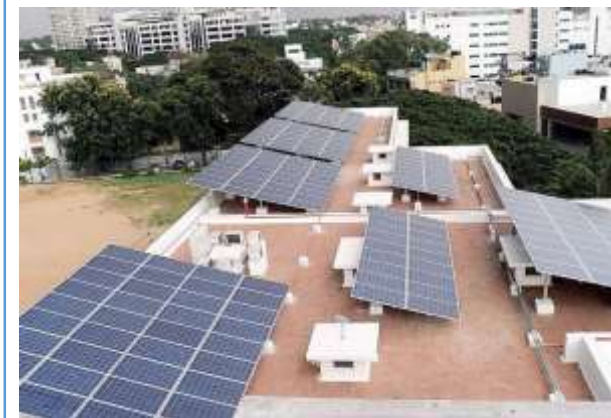
Installed Solar Panels at Surangi Unit, reducing 80 MT carbon emissions per month
