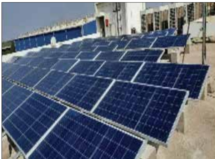
Solar panels were installed at Dahej site as part of your Company's sustainability efforts in energy saving.
