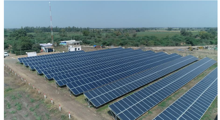
12.5 MW Solar plant installed at Bharuch
