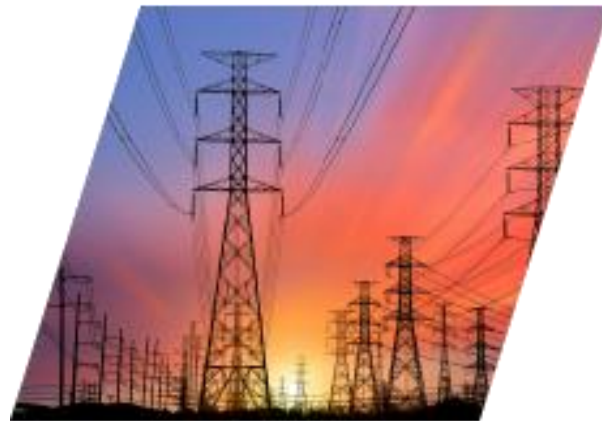
Power Transmission & Distribution
