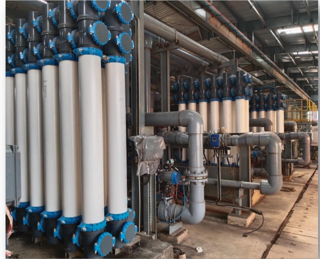
NMDC ZLD Plant, Chhattisgarh, India
