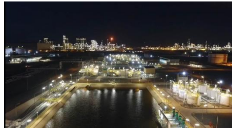
102 MLD Industrial Effluent Treatment Plant for PETRONAS, Malaysia Largest industrial Effluent Treatment Plant in South East Asia
