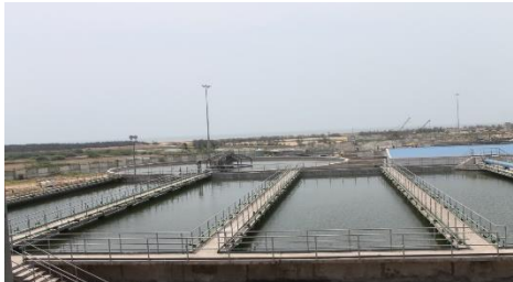
54 MLD Effluent Treatment and recycling plant, for Indian Oil Corporation Limited, Paradip, Odisha, India India's largest industrial water recycling plant
