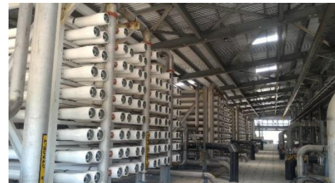
50 MLD BWRO (Desalination), for Reliance Industries, Dahej, India Turnkey project executed in record 8 months 24 days
