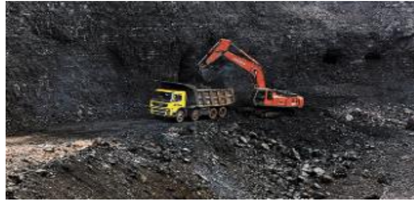
Coal Mines (Total Capacity of 2.04 MMT p.a.)
