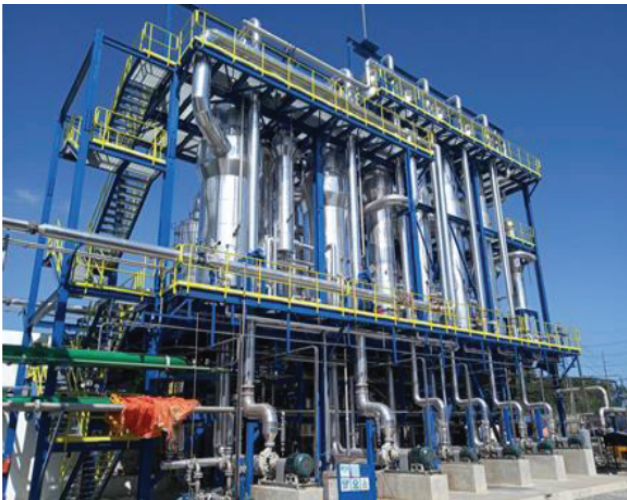
Praj successfully handed over a biomethanated vinasse pre-treatment & evaporation plant, & modernized distillery plant in Dominican Republic.
