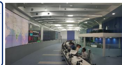
Operations & Maintenance Command & Control Center (OMCCC)
