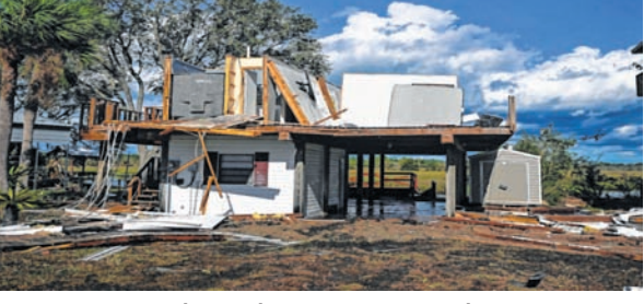
A destroyed house is seen in Keaton Beach, Florida on Wednesday after Hurricane Idalia made landfall
