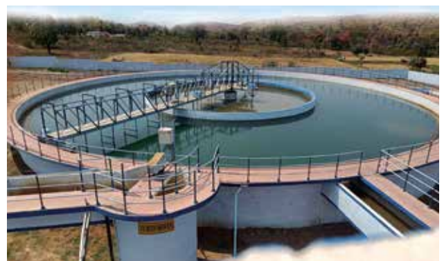
29.10 MLD Water Treatment Plant for Indwar Multi village Rural water Supply Scheme, in Madhya Pradesh.
