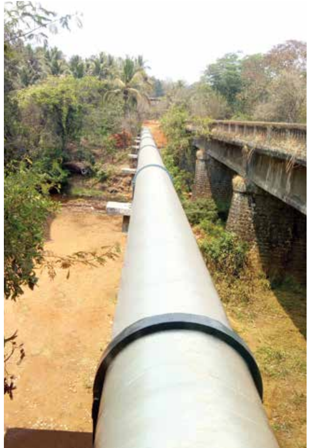
1200 mm dia MS pipeline laying for Tillari Water Supply Project for Maharashtra Jeevan Pradhikaran, in Maharashtra
