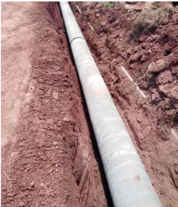
600 mm dia. BWSC pipeline laying for Tillari Water Supply Project for Maharashtra Jeevan Pradhikaran, in Maharashtra
