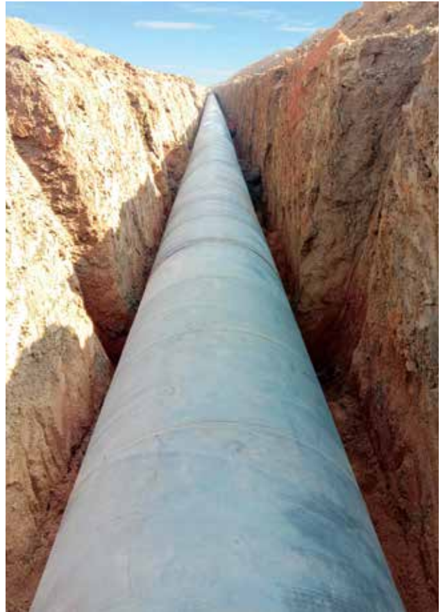
1500 mm dia MS Pipeline laying work for Bilaspur Water Supply Scheme, in Chhattisgarh.
