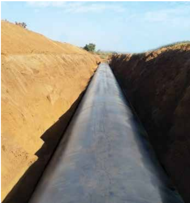
2028 mm dia MS pipeline laying work for Narmada Water Resources, Water Supply Scheme & Kalpsar Department, Palanpur in Gujarat.
