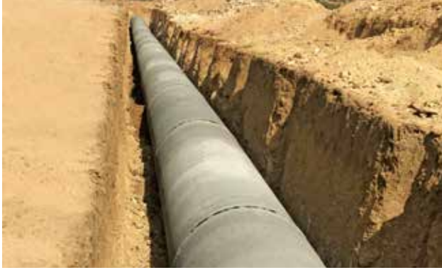
1700 mm dia PCCP pipeline laying for KPCL Bellary Thermal Power Plant, in Karnataka
