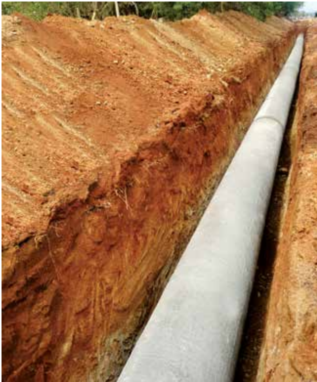
1067 mm dia MS pipeline laying for Madurai Water Supply Scheme, Madurai, in Tamilnadu.
