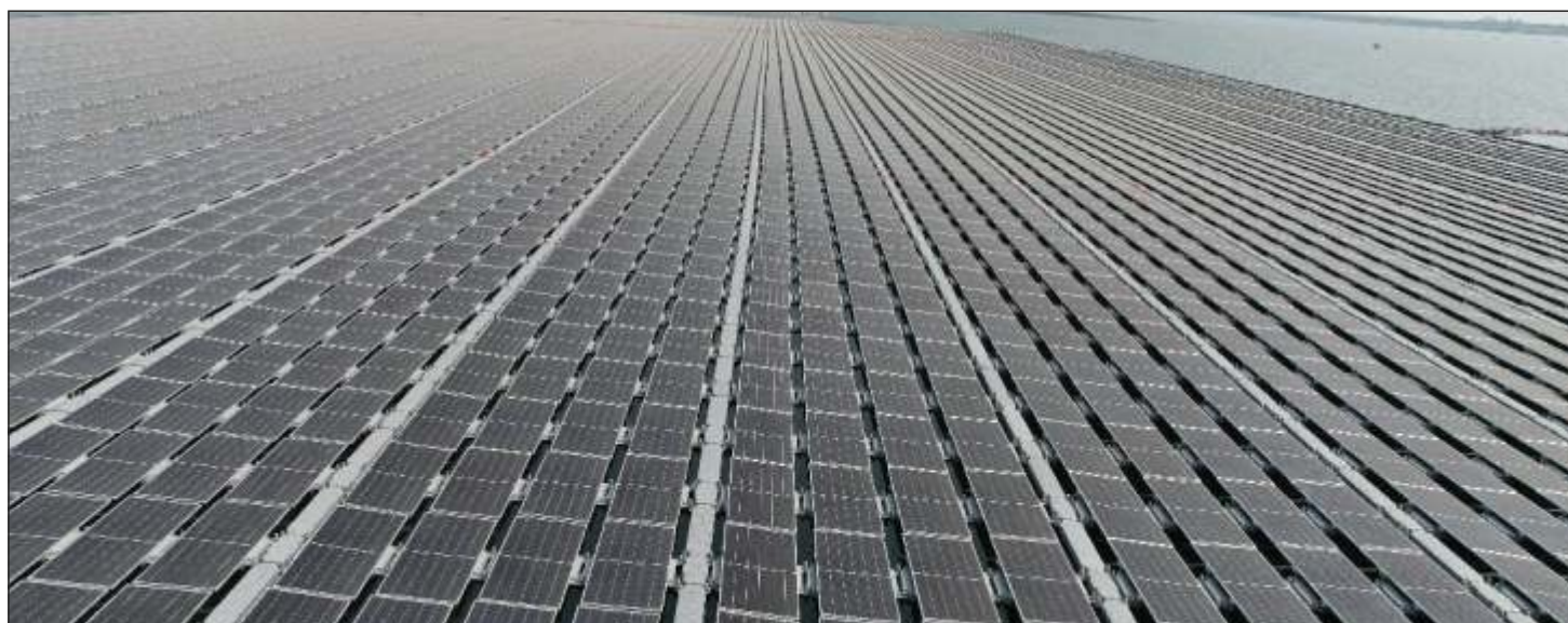
IREDA funded 100 MW Floating Solar Power Project of M/s. AMP Green Energy Seven Pvt. Ltd., located at Omkareshwar Reservoir, in Khandawa Dist. Madhya Pradesh.
