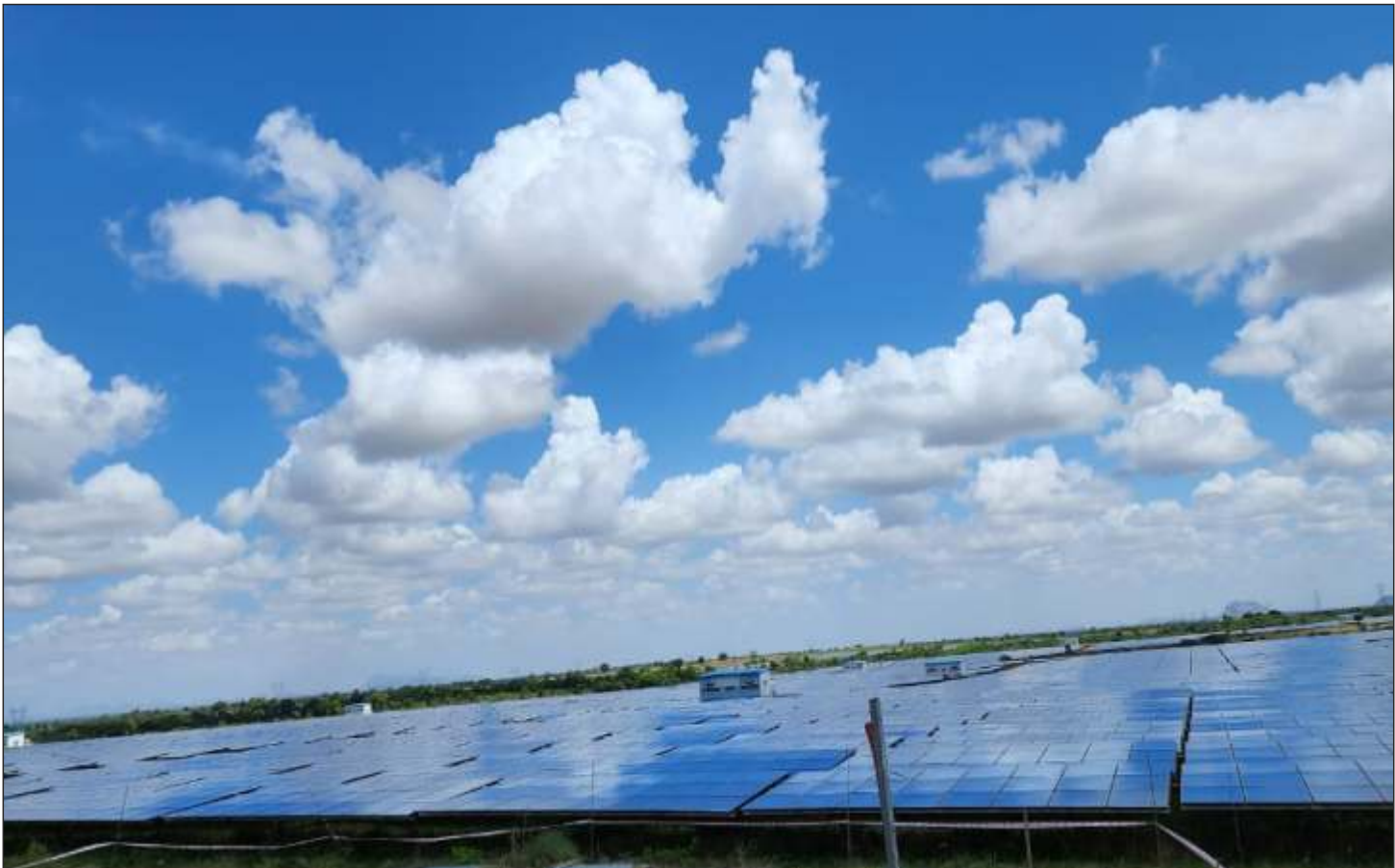
IREDA funded 50 MW / 50.49 MWp Solar Power Project of M/s. ACME Group located at Anantapur District, Andhra Pradesh.
