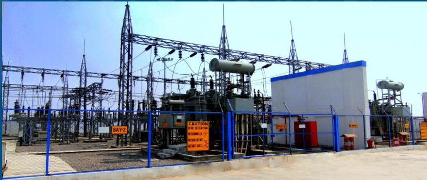
Tata Power - HT Substation
