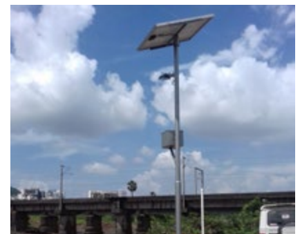
Installed Solar Street Light in Panvel
