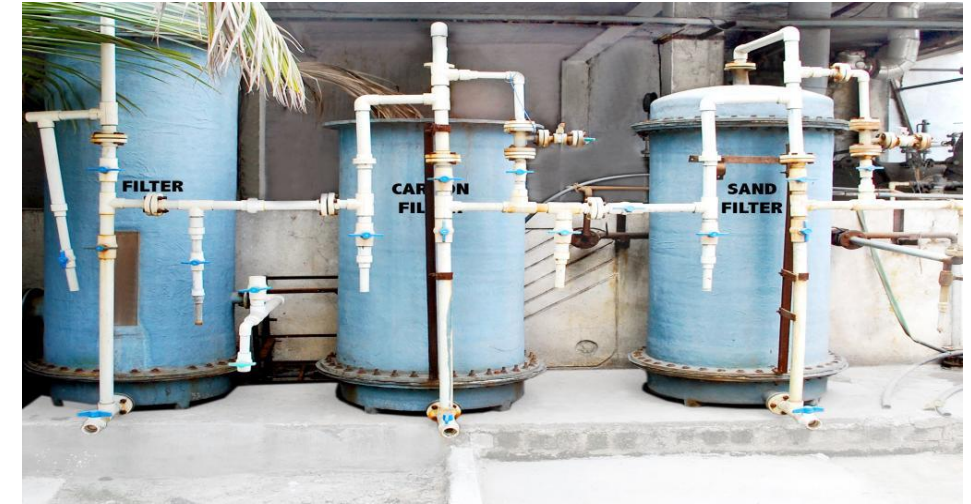
(Reverse Osmosis Plant) R.O. Plant
