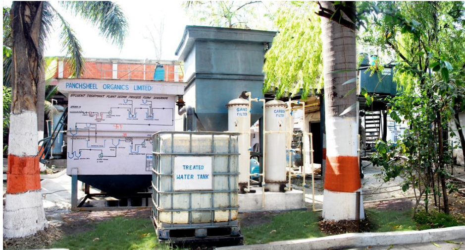
Effluent Treatment Plant
