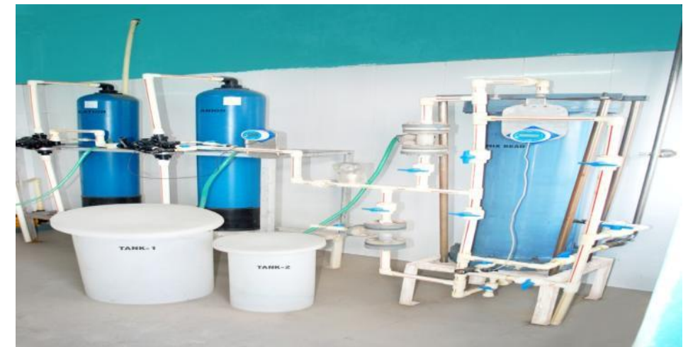
(De-mineralised Water Plant)
