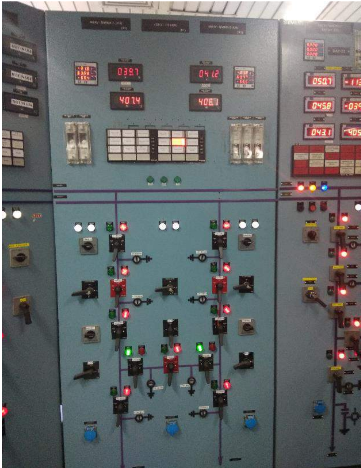
400/220 kV PGCIL substation at Jalandhar – indicating Voltage, Phase current and Power
