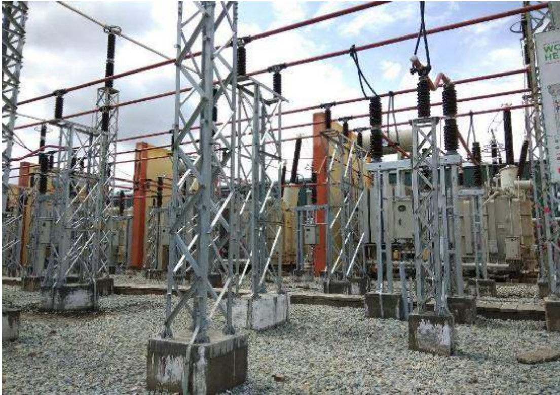
Inter – Connecting Sub – station yard
