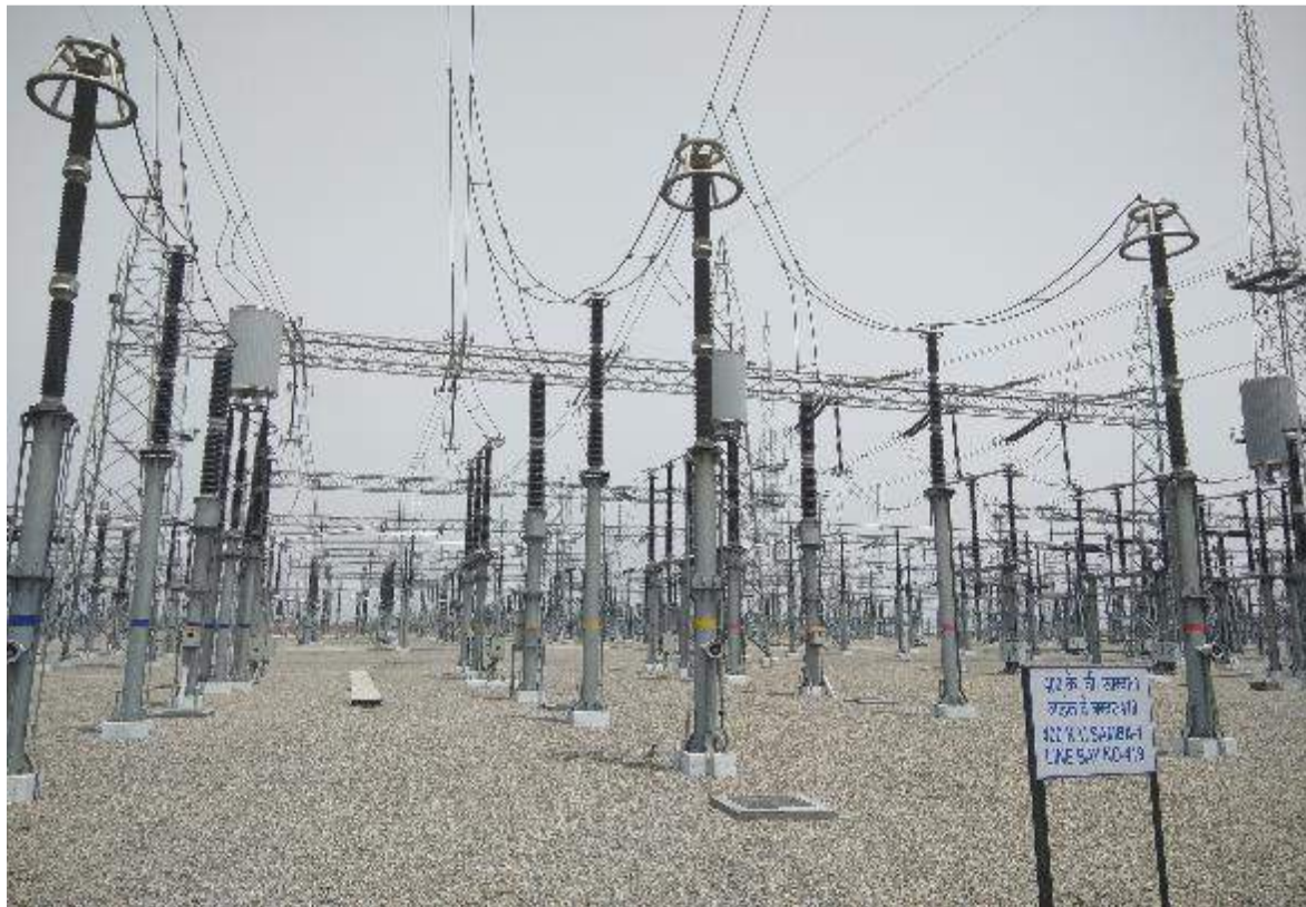
400/220 kV PGIL Substation at Jalandhar Samba Line 1 Bay
