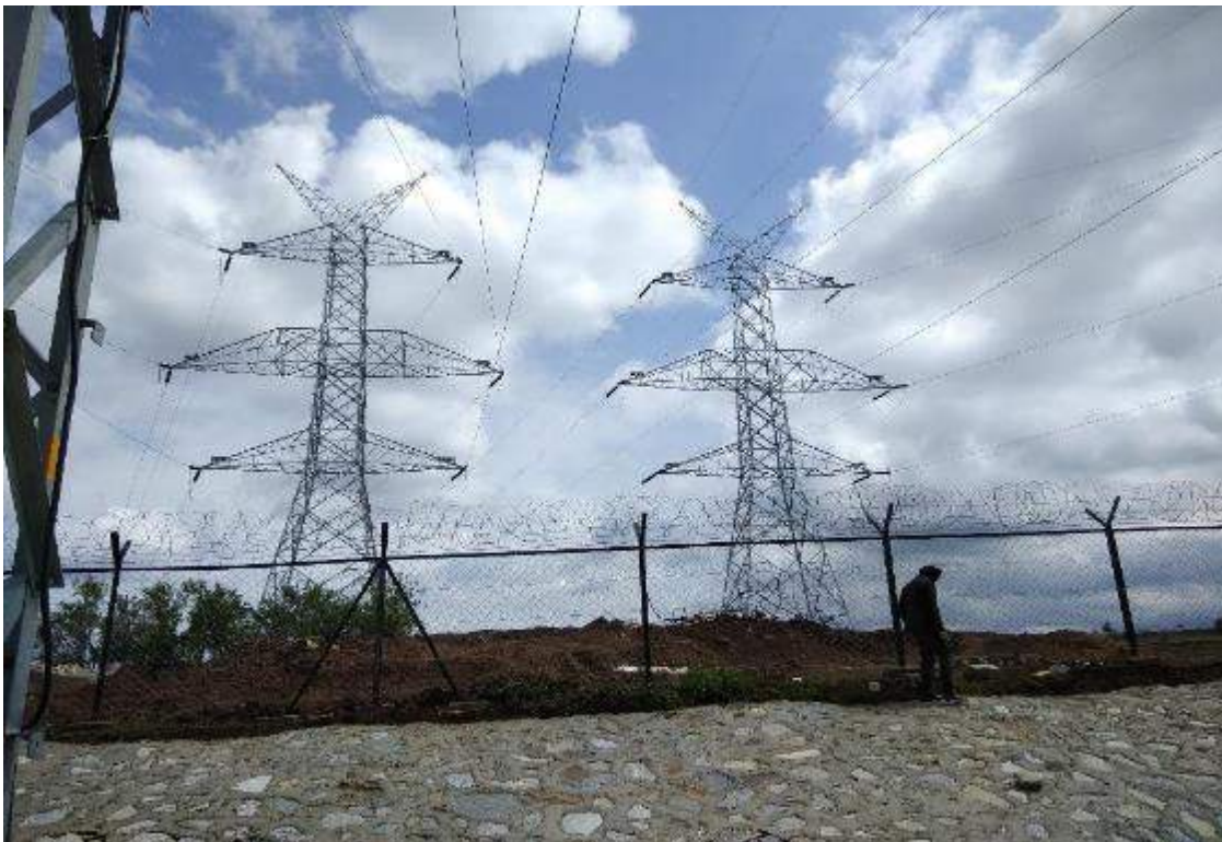
220 kV outgoing transmission lines
