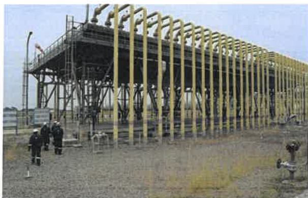
CS - 1 Gas After Cooler
