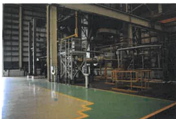
CS - 1 Compressor Station
