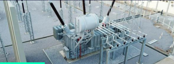
High Voltage Power transformers
