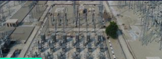
High Voltage Substations, AC & DC
