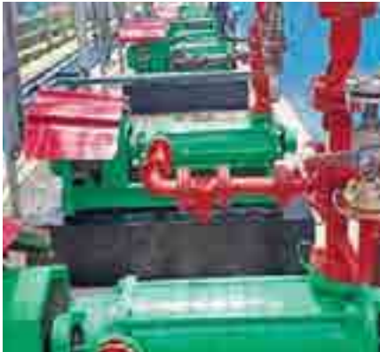
Conventional Pump seals are replaced with Mechanical seals which ensures no leakage and spillage free dykes.
