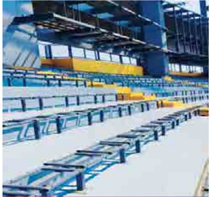
Renowned Stadium Rehabilitation work completed in record 60 days, of stands and structures, with Pro Polyshield UV 75 and BR PU High Gloss Enamel.
