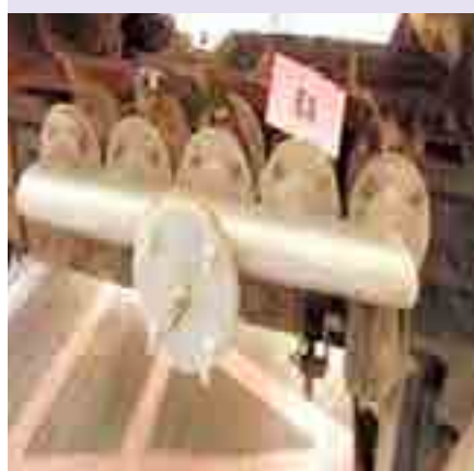
Color coded QC approval sticker on the tanker unloading valve
