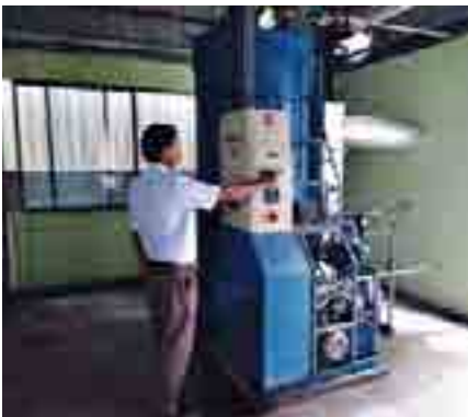
Condensate Recovery System for recovering water from steam
