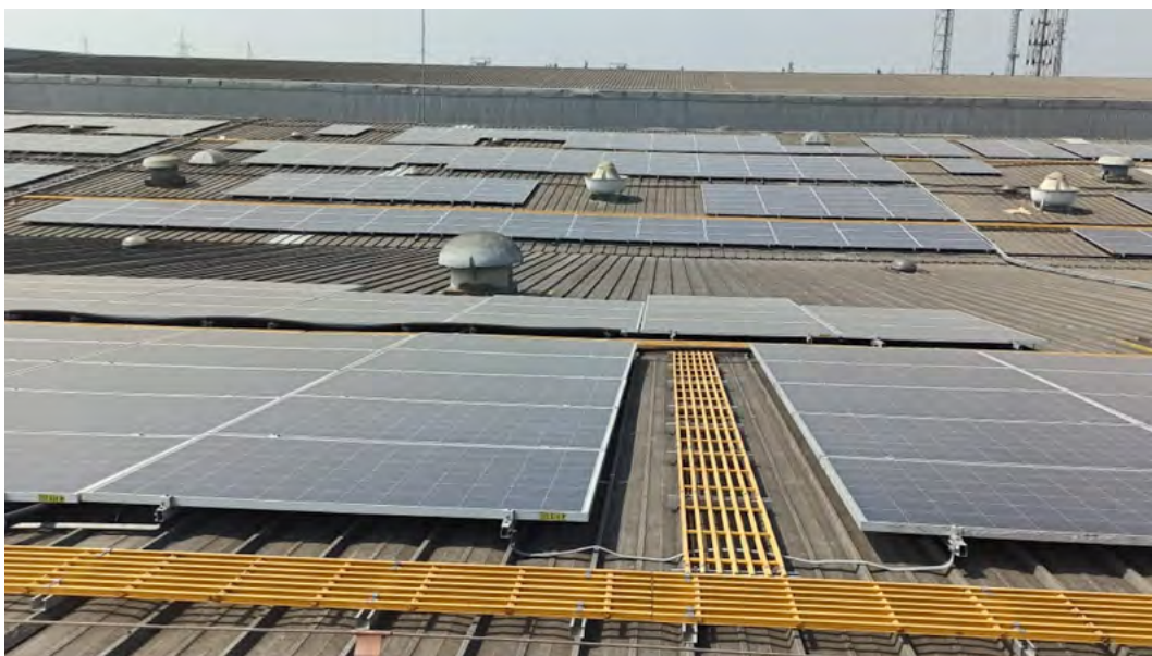
Rooftop Solar Plant at Pantnagar
