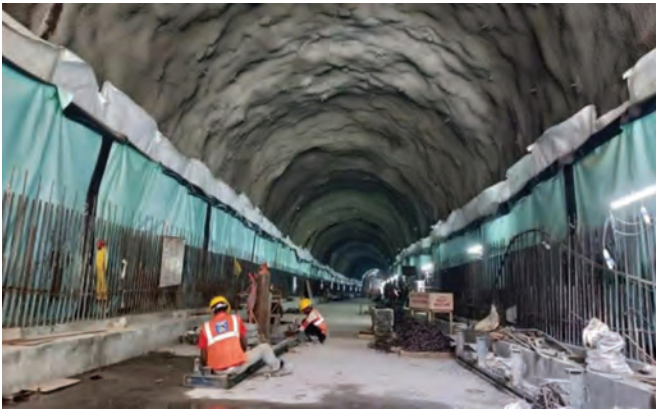
The Mumbai Metro line 3, currently under construction, will be the first underground line of the city. The Construction Chemicals business is supplying MasterSeal 700BG, a PVC synthetic waterproofing membrane for the establishment of complete watertight construction of the underground metro rail twin NATM tunnels.
