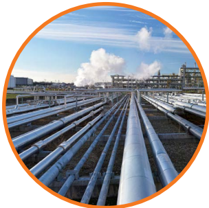
Gujarat Gas Limited Project-Gas distribution Products Used-Pipes
