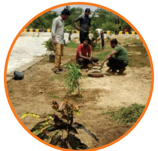
BSES Yamuna Power Limited Project-Earthing Electrodes Products Used-GI Pipes & Pole
