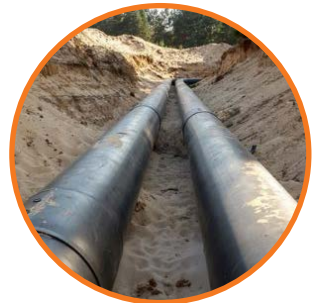
Jal Shakti Department Shimla Project-Water distribution Products Used-GI Pipes
