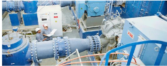
Pumping Station & Distribution
