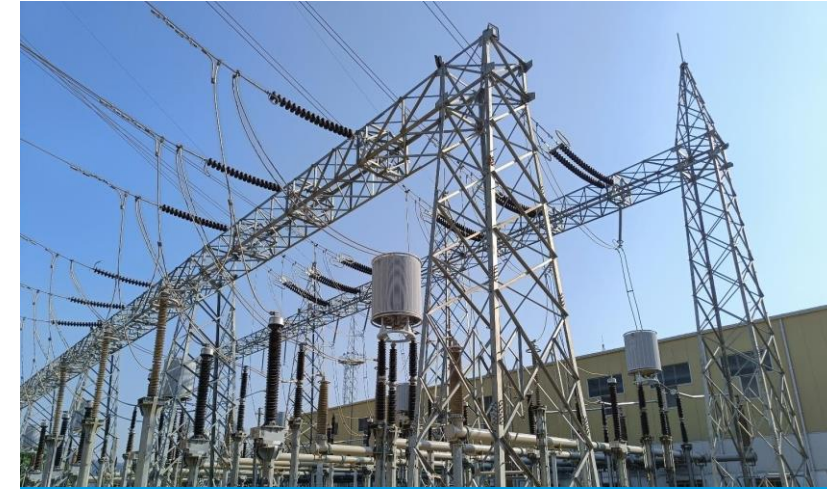
Jauljibi Substation, Uttarakhand
