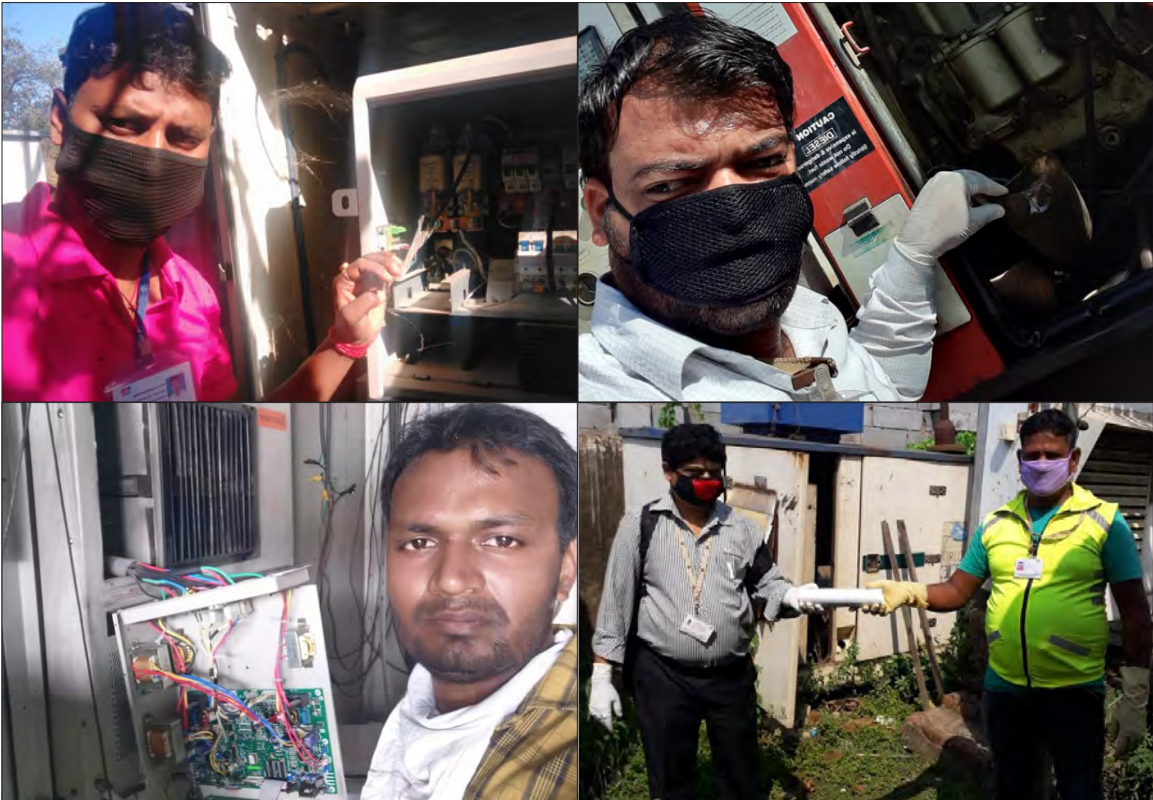
Best in Class O&M of Telecom Infrastructure.
