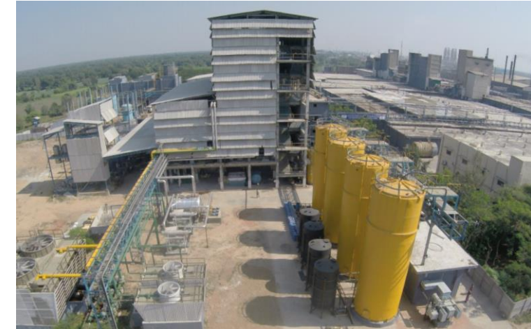
Multiple Effect Evaporator Plant (MEEP)
