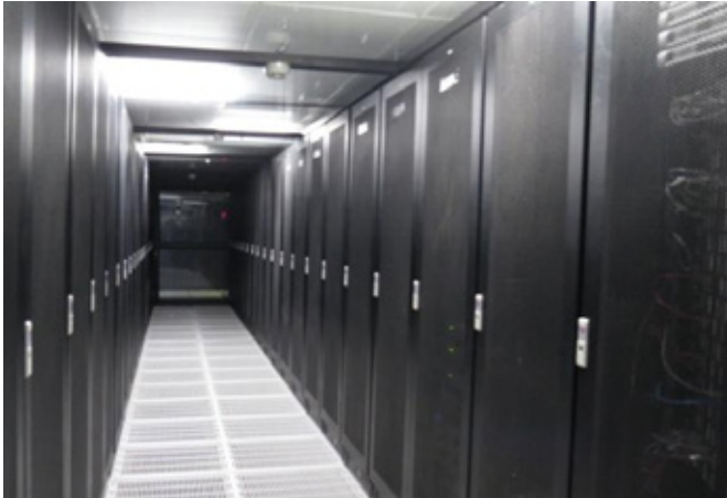
RailTel Data Center at Gurugram
