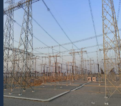
Adani(BKTL) at Khetri, Rajasthan - Charging of 80 MVAR Reactors & 765kV AIS line bays
