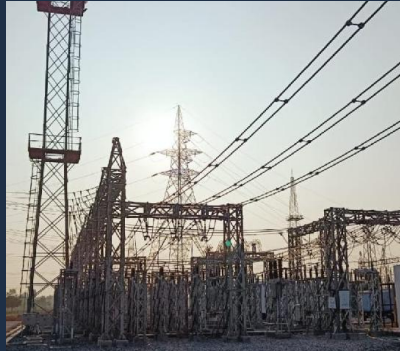
JUSNL, Meral, Jharkhand - Commissioning of 50 MVA Transformer along with 132kV & 33kV AIS associated bays
