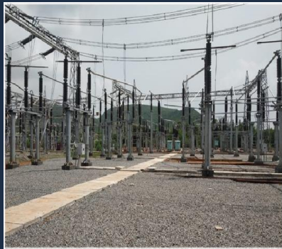
HPCL, Vizag, AP - 220kV AIS Bay extension at APTRANSCO Kalpakka site
