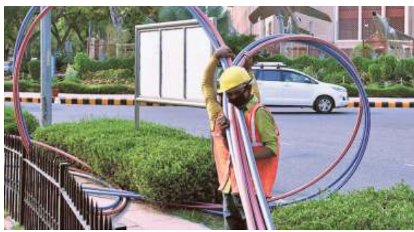
DoT has indicated that it is willing to foot the entire capex to maintain, rebuild and service the network. KAMAL NARANG
