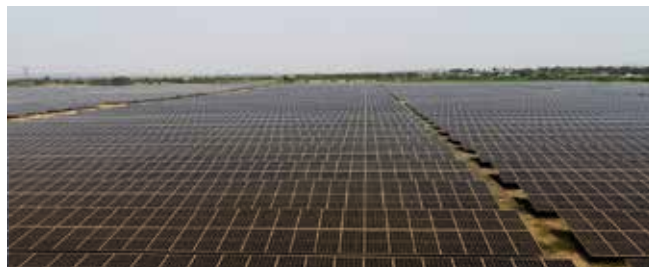
This image represents the first captive solar power plant of 20 MW over 60 acres in North Karnataka.
