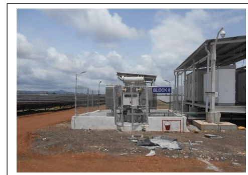
View of the solar power plant
