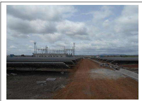
View of the solar power plant
