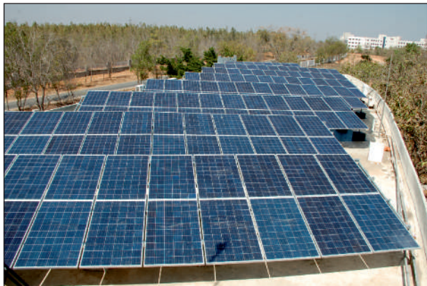
A view of BEML eco-friendly solar panels
