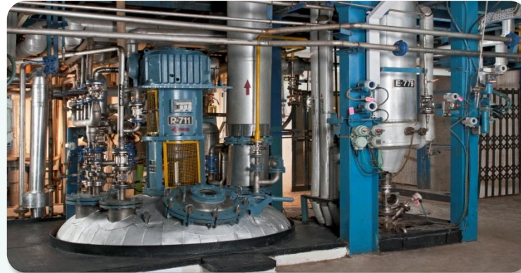
Agro Chemical Plant - Panoli
