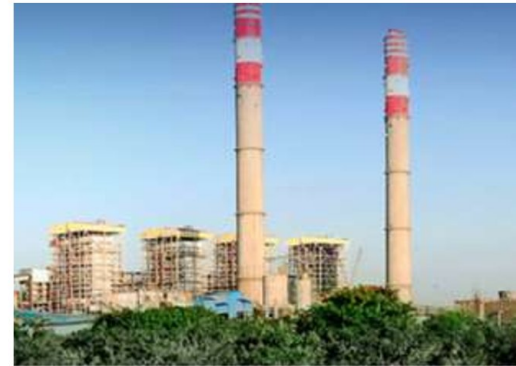
JSW Energy Ltd., Ratnagiri
