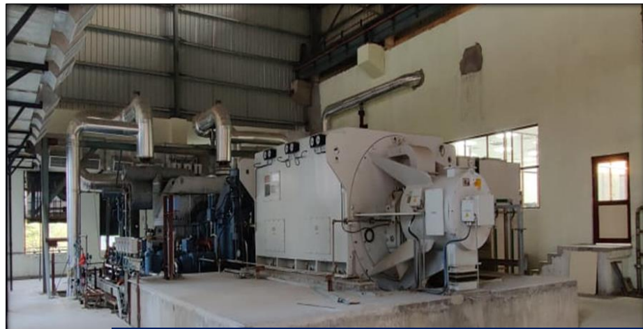
Steam Turbine Generator
